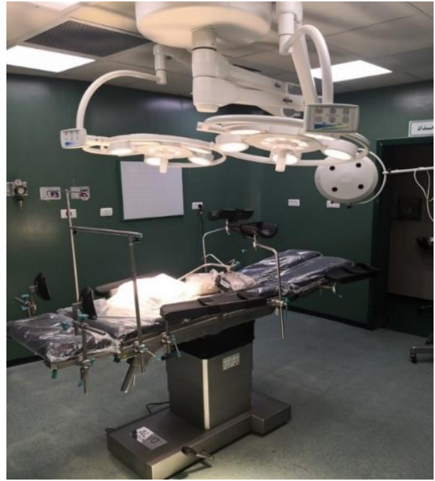
Figure 5: The installed ceiling operating light and operation table at Alshifa hospital in Gaza
